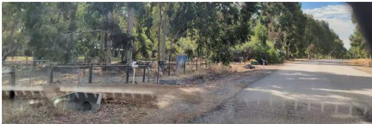
Figure 4 – Section 3 Insufficient Carriageway Offset
