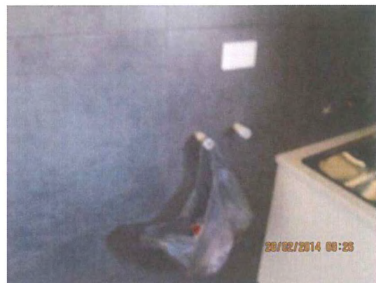
Washing Machine Plumbing
