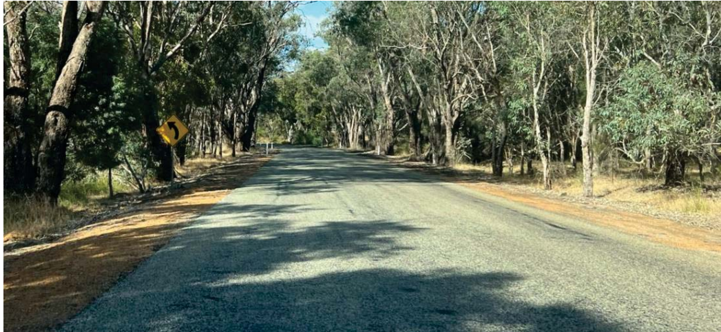
Photograph 2 – Typical layout of Blue Plains Rd (6m wide seal and gravel shoulders of various widths)
