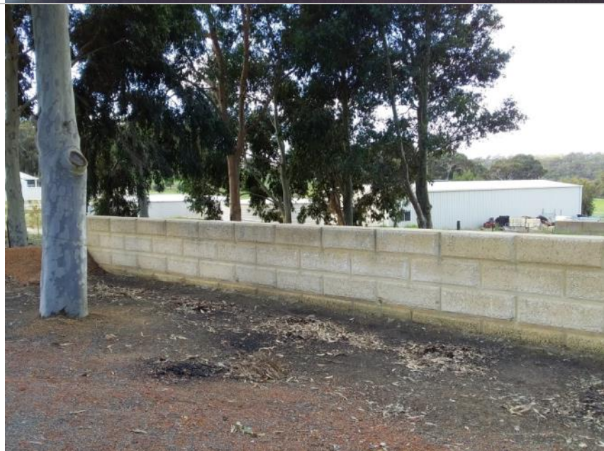
Photo 2: Front limestone wall (looking north) at Holstein Loop, Lower Chittering (Planning Officer, 2019)
