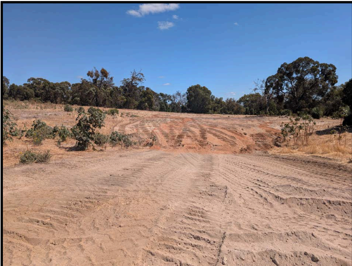
Image 4: Example of 'Open Pit' being filled in by landowner (Senior Planning Officer, March 2026)
