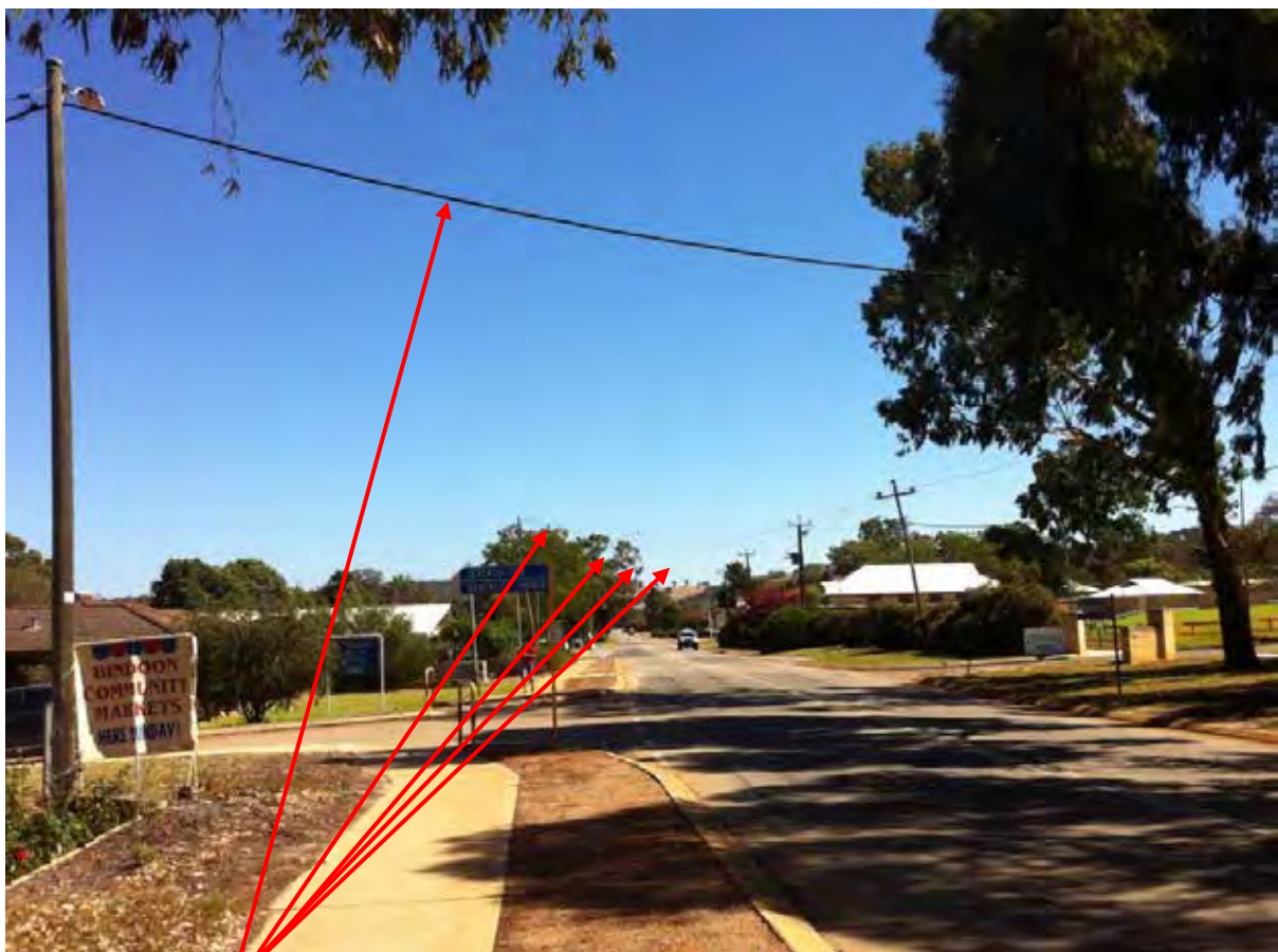
Power lines crossing GNH in front of Community Health Clinic
